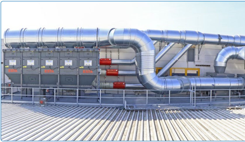
The extraction system is installed on the roof of the hall.
